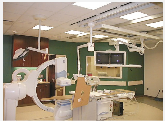
Unistrut Medical Equipment Support
