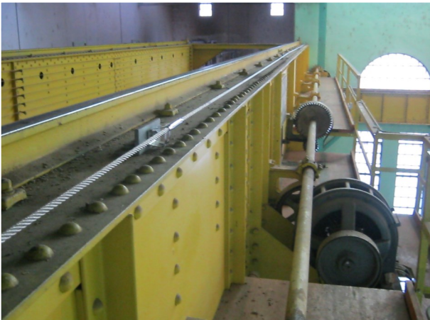
Engineered fall protection system inside dam turbine house
