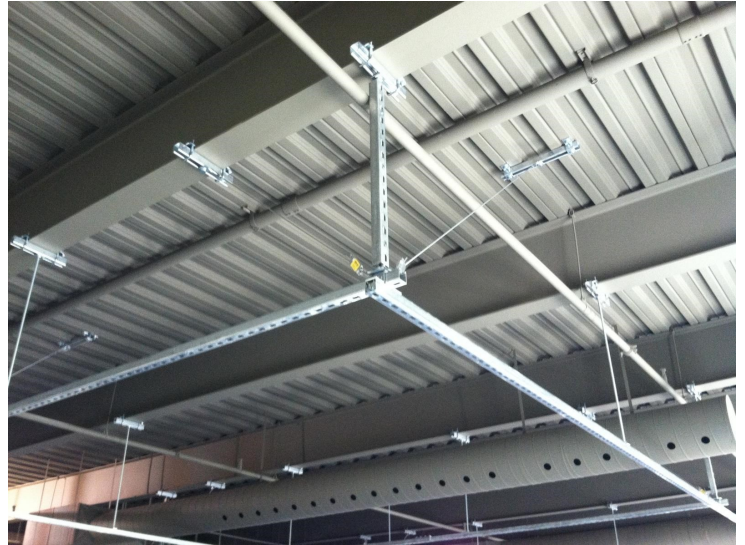
Unistrut grid braced with Gripple seismic cable
