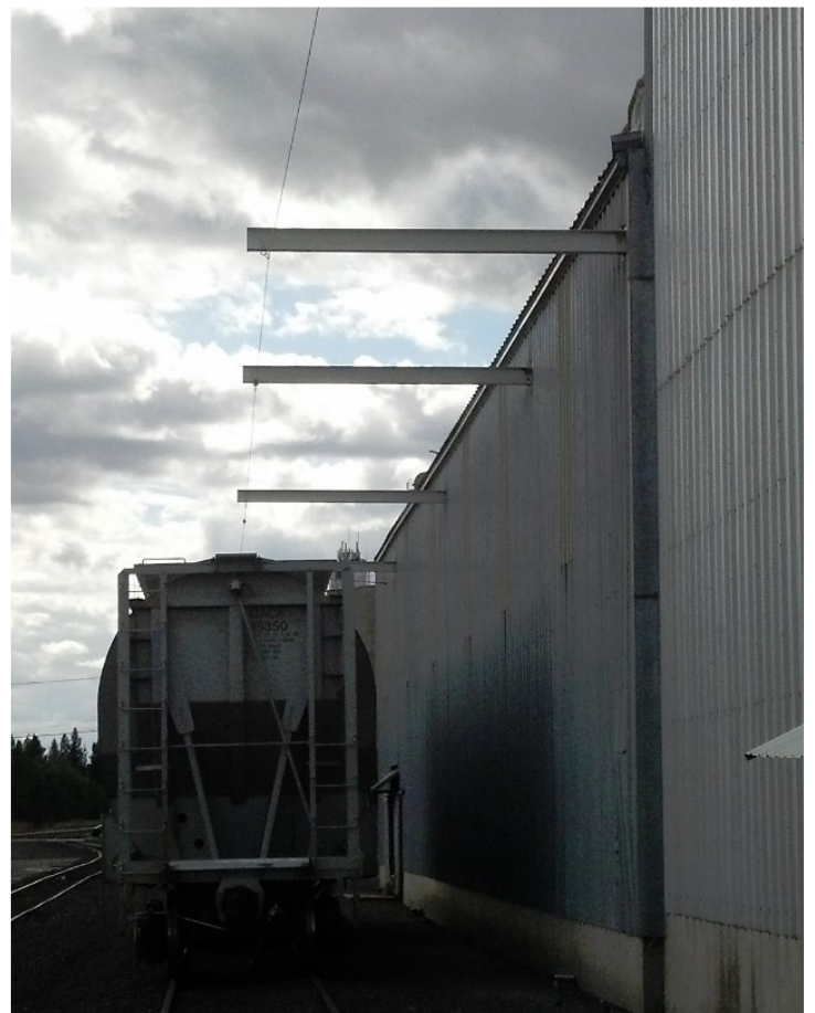
Railcar fall protection systems
