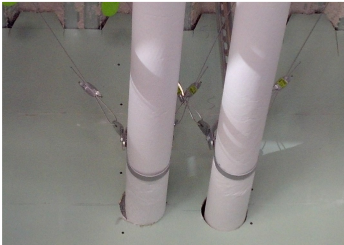
Gripple cable bracing pipe
