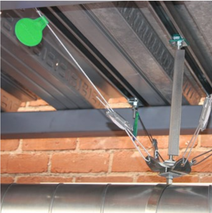
Gripple and Unistrut seismic bracing
