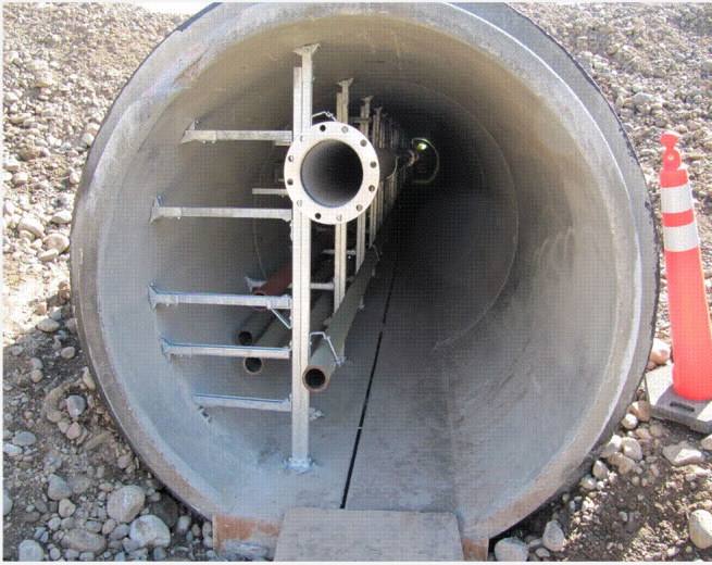
Unistrut in underground pipe/utility tunnel
