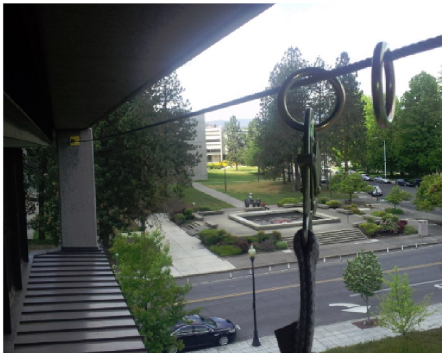
Horizontal lifeline on building exterior
