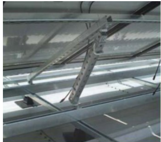
Solar Rooftop Support with Unistrut & Telespar
