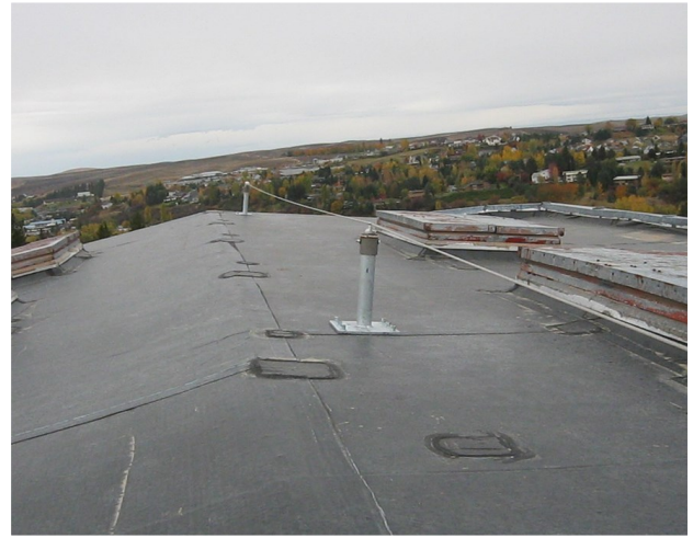
Rooftop horizontal cable systems
