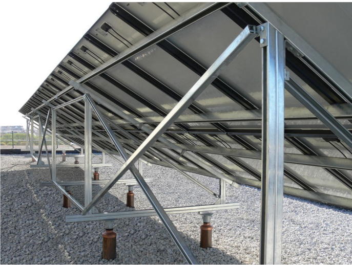
Solar Panel Framing
