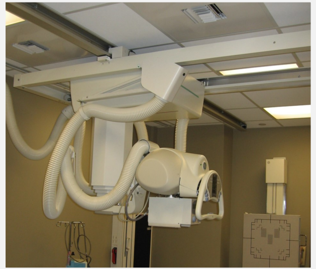
Finished X-Ray system Hanging from unseen Unistrut
