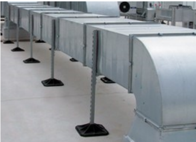
Rooftop ducting H-Frame supports
