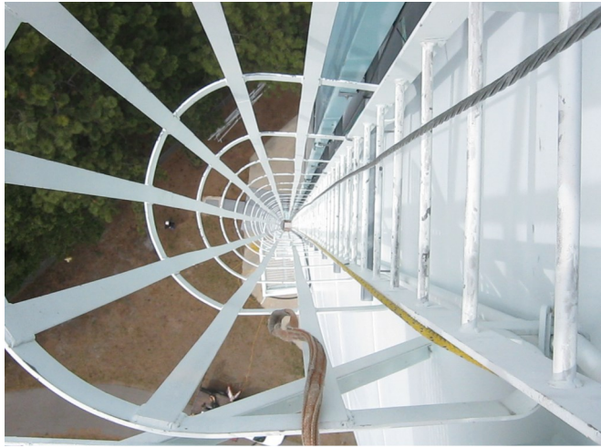
Ladder cable safety systems
