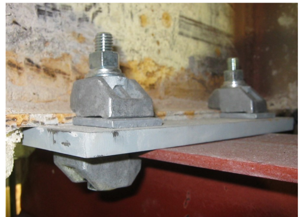
Example of installed girder clamps in hospital
