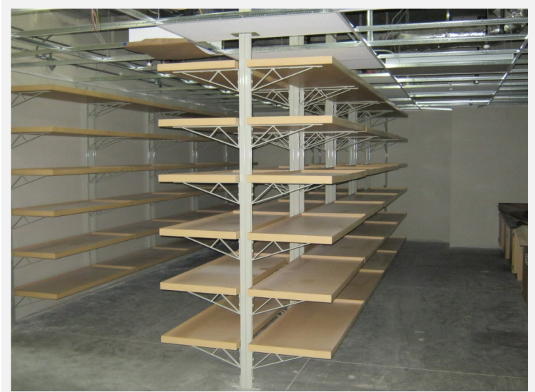
Island and wall shelving with base secured to concrete floor
