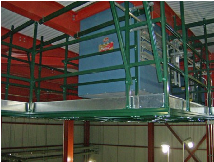
Unistrut frame & grating suspended from overhead structure to access mechanical equipment
