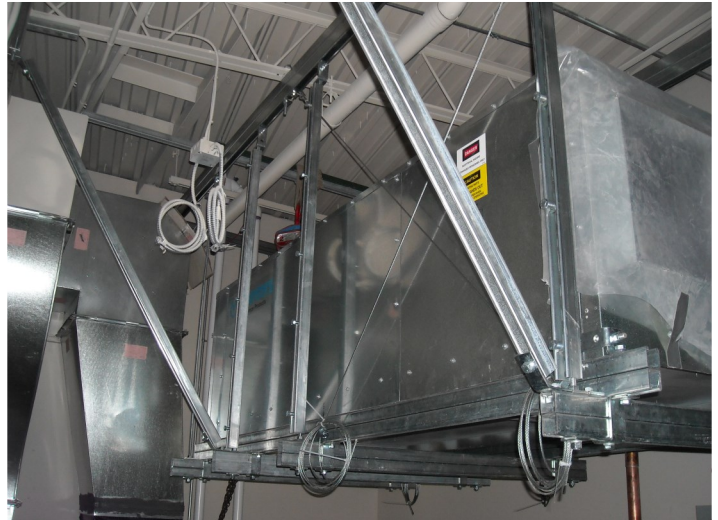
Heat pump support with seismic bracing
