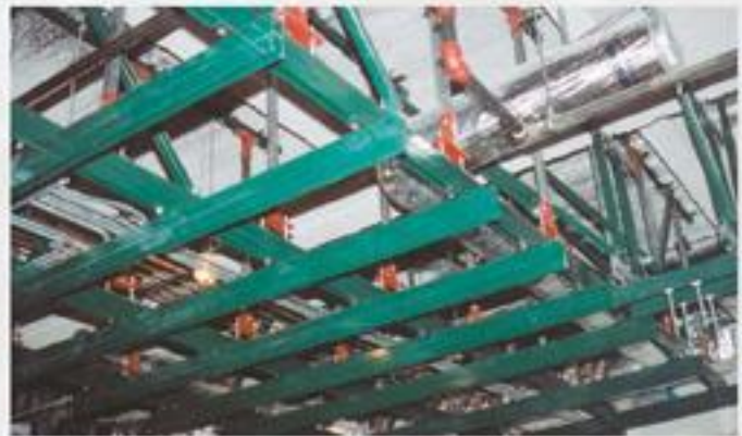
Multi-rail support system with Telespar drops.
