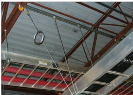
Bracing of electrical services
