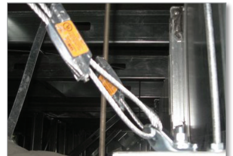
Bracing of rectangular ductwork
