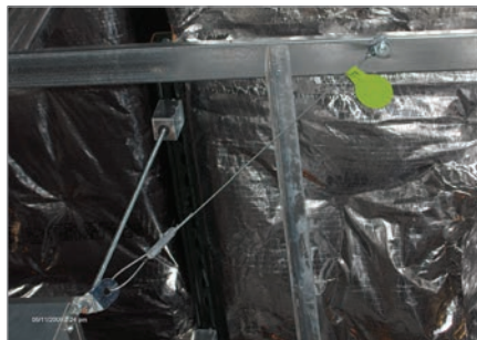
Bracing of busduct
